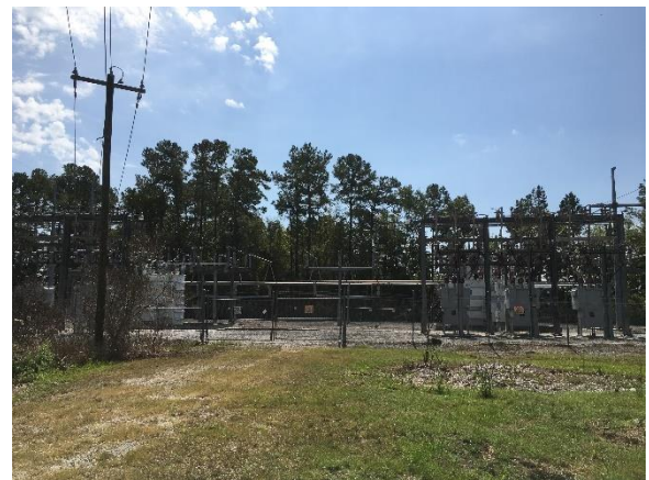
Electrical substation south of site.
